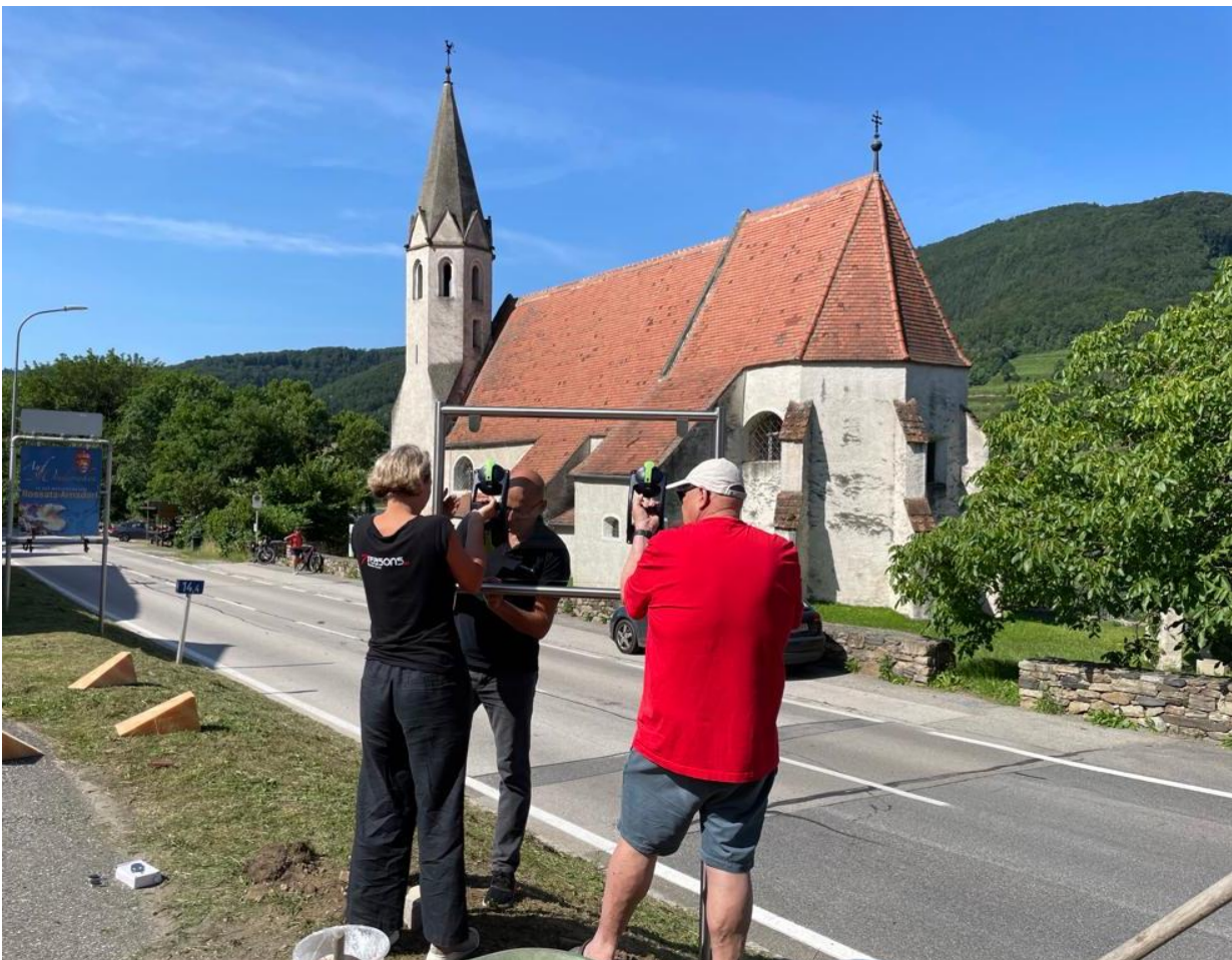
St. Johann im Mauerthale, installing the frame of the "trompe-l'oeil". Cooperation between workers of the municipality of Rossatz-Arnsdorf, the company 7reasons and local supporters.
