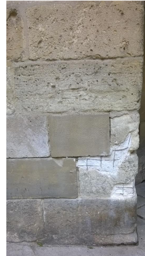
Inappropriate repair, lack of knowledge.
