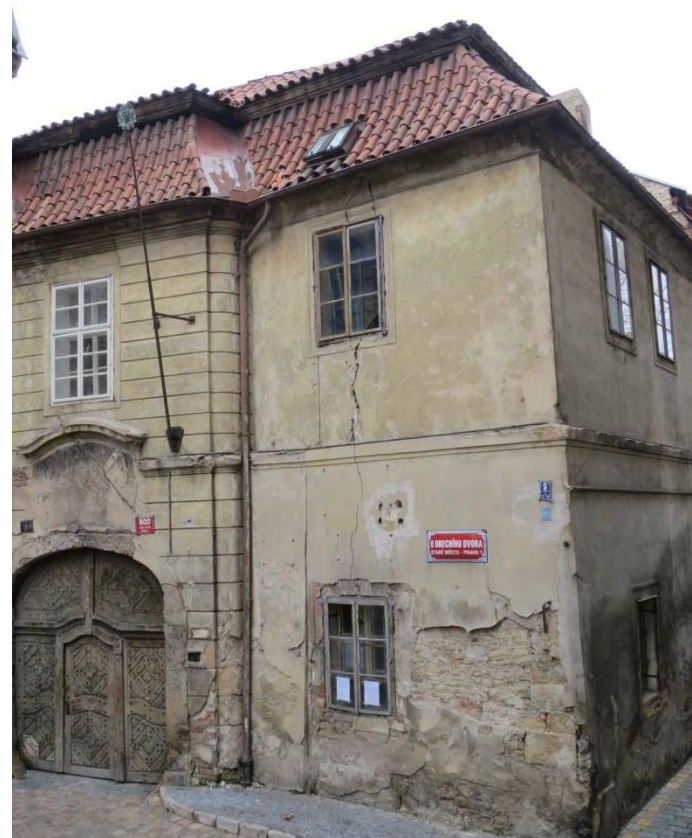
Lack of maintenance, property issues.
